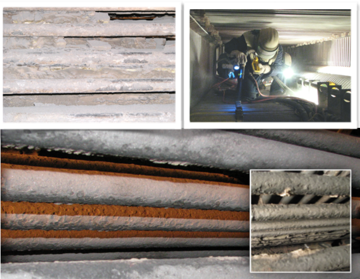
Deep pitting observed in biomass boiler superheater tubes after abrasive blasting to remove slag deposit. Photo by Furnace Mineral Products Inc.
