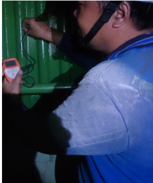
Quality control testing following the application of ceramic coating in a pulp and paper plant CFB boiler in Asia, Photo by Furnace Mineral Products Inc.
