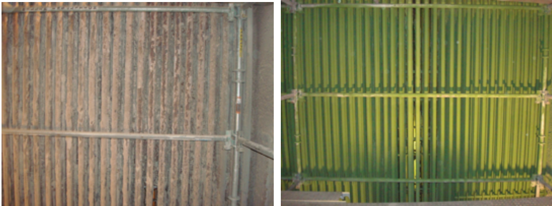
a. Complete blockage of superheater tubes. b. Application of ceramic coating to extend boiler uptime by reducing forced cleaning outages.
