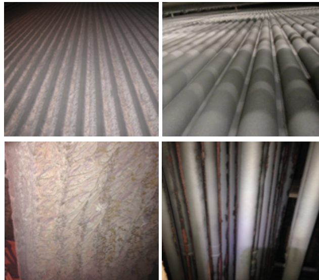
Dry abrasive blasting to remove slag build up from boiler tube surface
