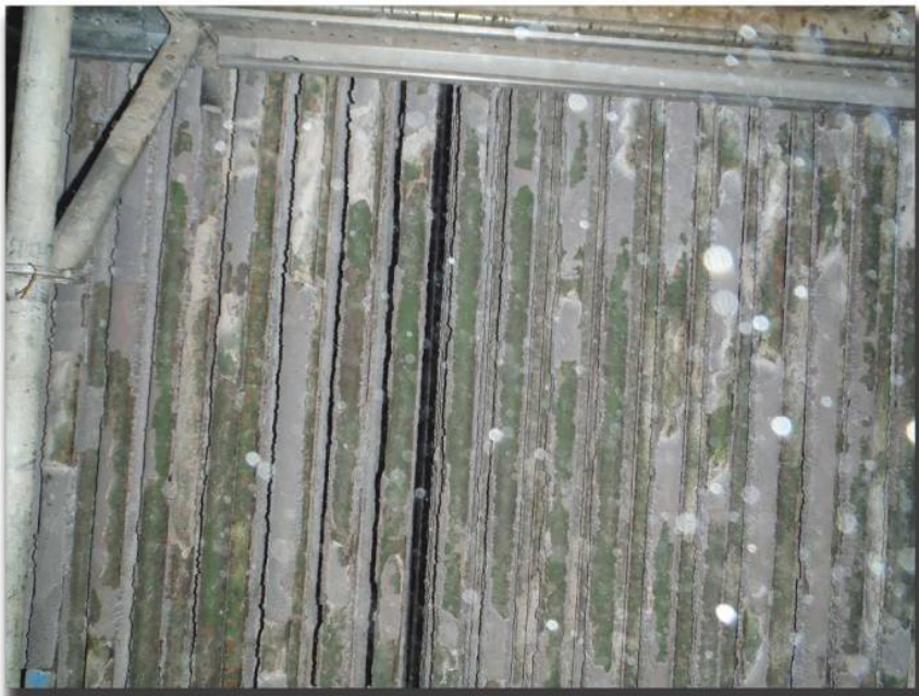
Coated superheater tubes are shaken to remove slag. Underneath the slag, the green ceramic coating is visible. Photo courtesy of Dan Gray, Rosebud Operating Services.
