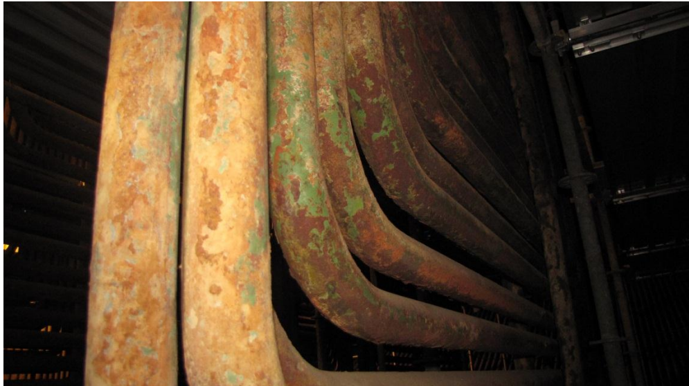
Figure 3: Patches of loosely adhered slag on coated superheater element is as found condition
