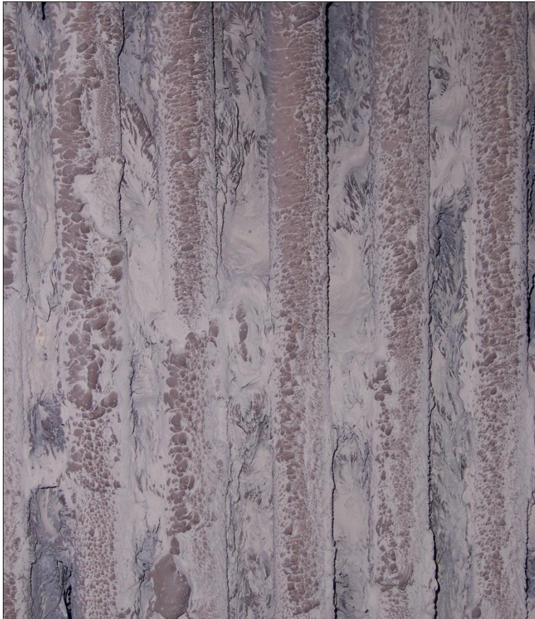
Figure 5: Plugged section of superheater prior to cleaning and ceramic coating application
