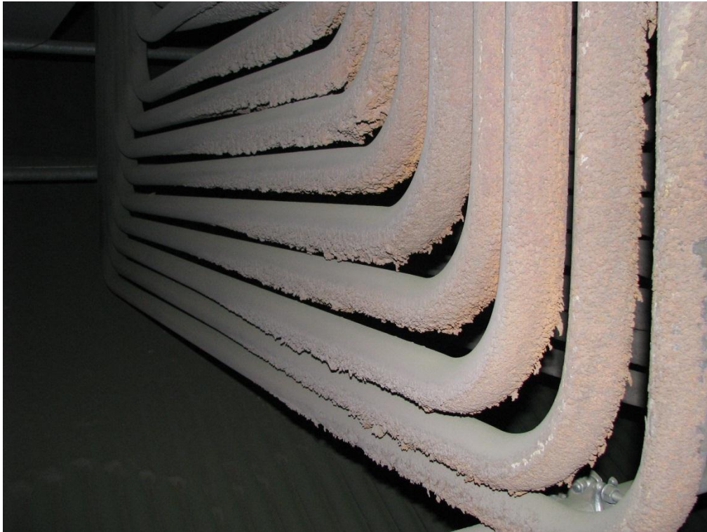
Figure 4: Heavy, well adhered slag on uncoated superheater element
